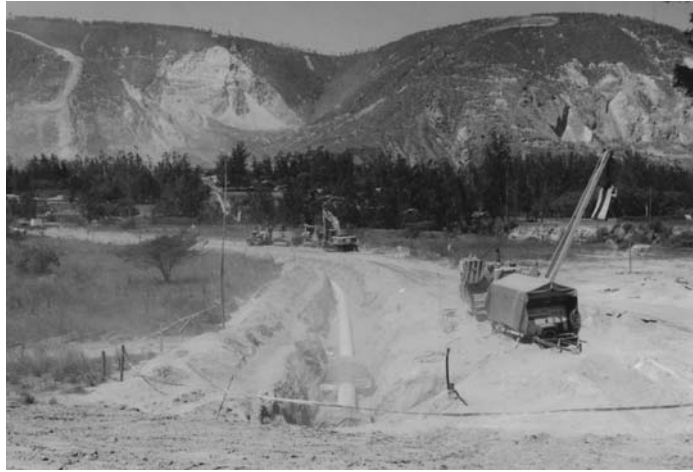
FIGURE 13: In 2001, a multinational oil consortium began construction on a second trans-Ecuadorian pipeline. The OCP pipeline travels 500 kilometers (312 miles) from the Amazon, over the Andes Mountains, to the Pacific Coast. Here in 2002, the underground pipeline is laid in the arid Andean zone north of the capital Quito. In the left corner, the buried pipeline cuts a trail down the slope.
